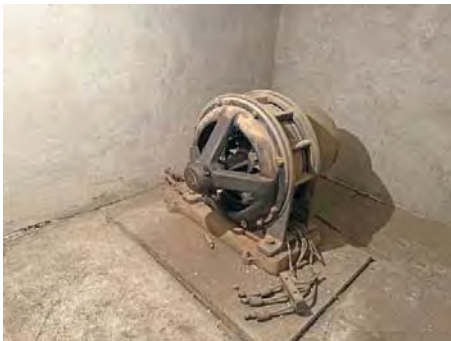
Basement Level Electric Motor Located in Basement of Main Mill.jpg
