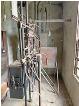
Main Mill Electrical Works Looking East.jpg
