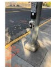
Substandard Pedestrian Signal Equipment
