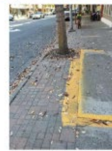
Failing Sidewalk due to Tree Roots
