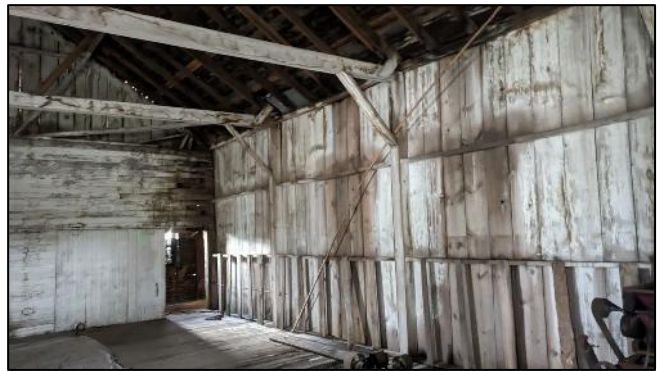
Photograph 12: View of the flour storage warehouse on the west side of the mill building.
