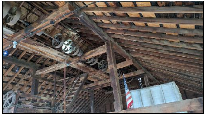
Photograph 10: View of the wheels that supported belts to operate machinery in the mill.
