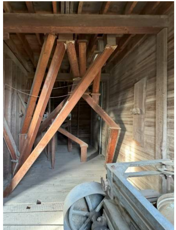
Equipment Room Small Chutes facing north.
