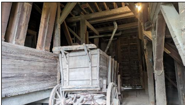
Photograph 5: View of the former loading area on the east side of the mill building.
